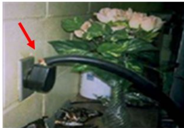
Cable has been pulled out of the plug end exposing internal wiring.
