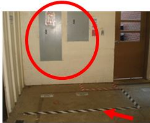
Building's Electrical Service Panels are taped off to keep free from obstructions.
